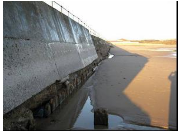
Littlehaven – Exposed timber foundations
